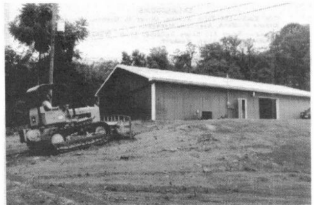
Grading was completed around the storage building which will remain with NCC, Inc.
